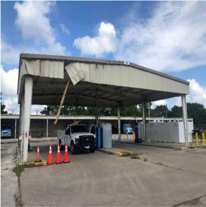
Canopy Before Repair
