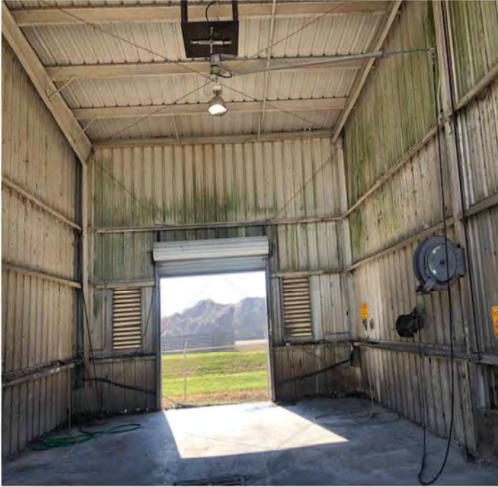
Wash Bay Before Repair
