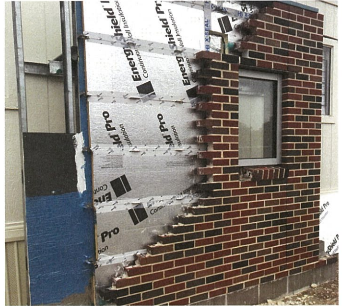
Flintco created a brick mock up for the Prairie View A&M University Public Safety Building.
