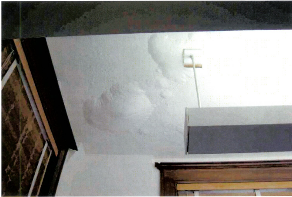
Rm 124: Moisture damage to plaster ceiling below mechanical room.
