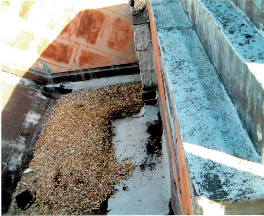
North roof gable drains. Water collects from backed up drain, sits against copper walls and infiltrates roof.
