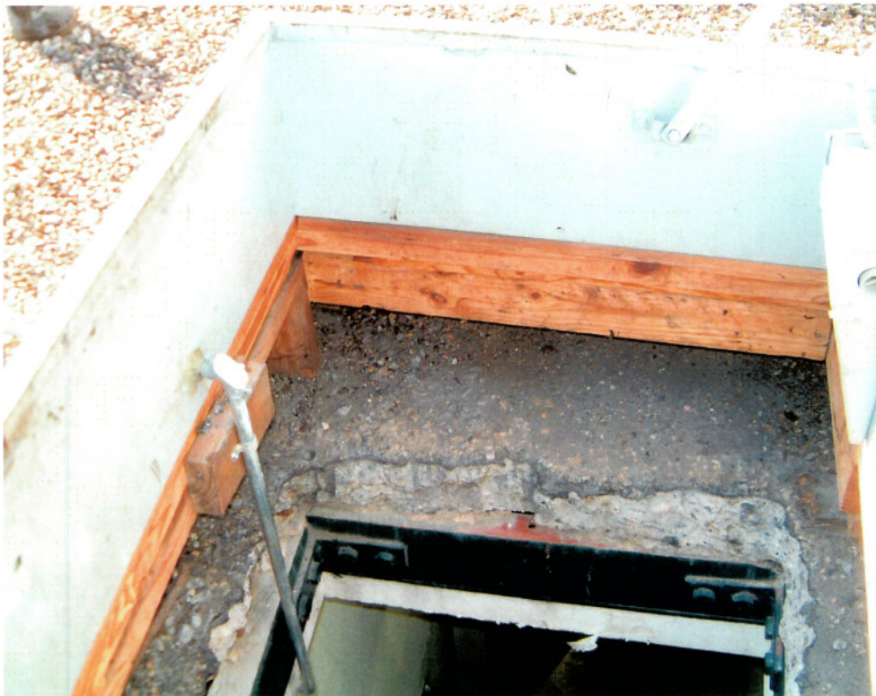
Concealed original roof under newer roof deck; Fire Hazard. Cinder concrete slab not visible to observe condition and monitor cracks.
