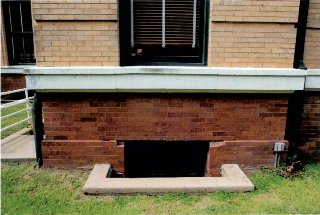
East Elevation: Spawling at Basement Window Lintel, Displaced Water Table, light well drain clogged.
