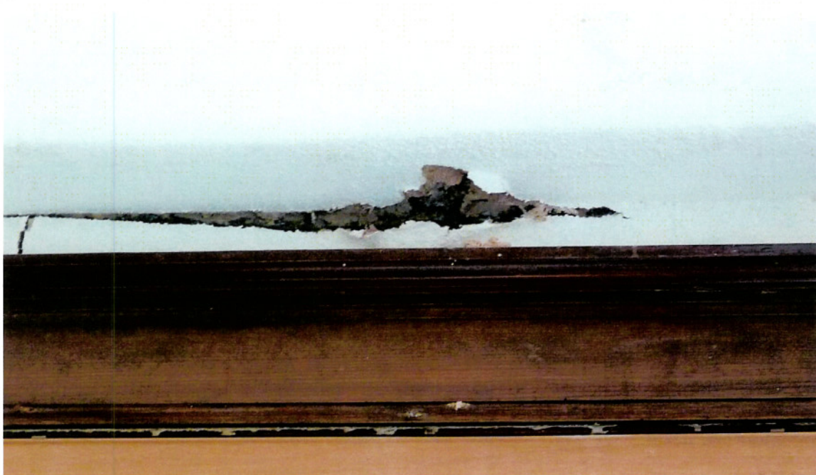
Plaster ceiling separating from wall at third floor exterior wall.
