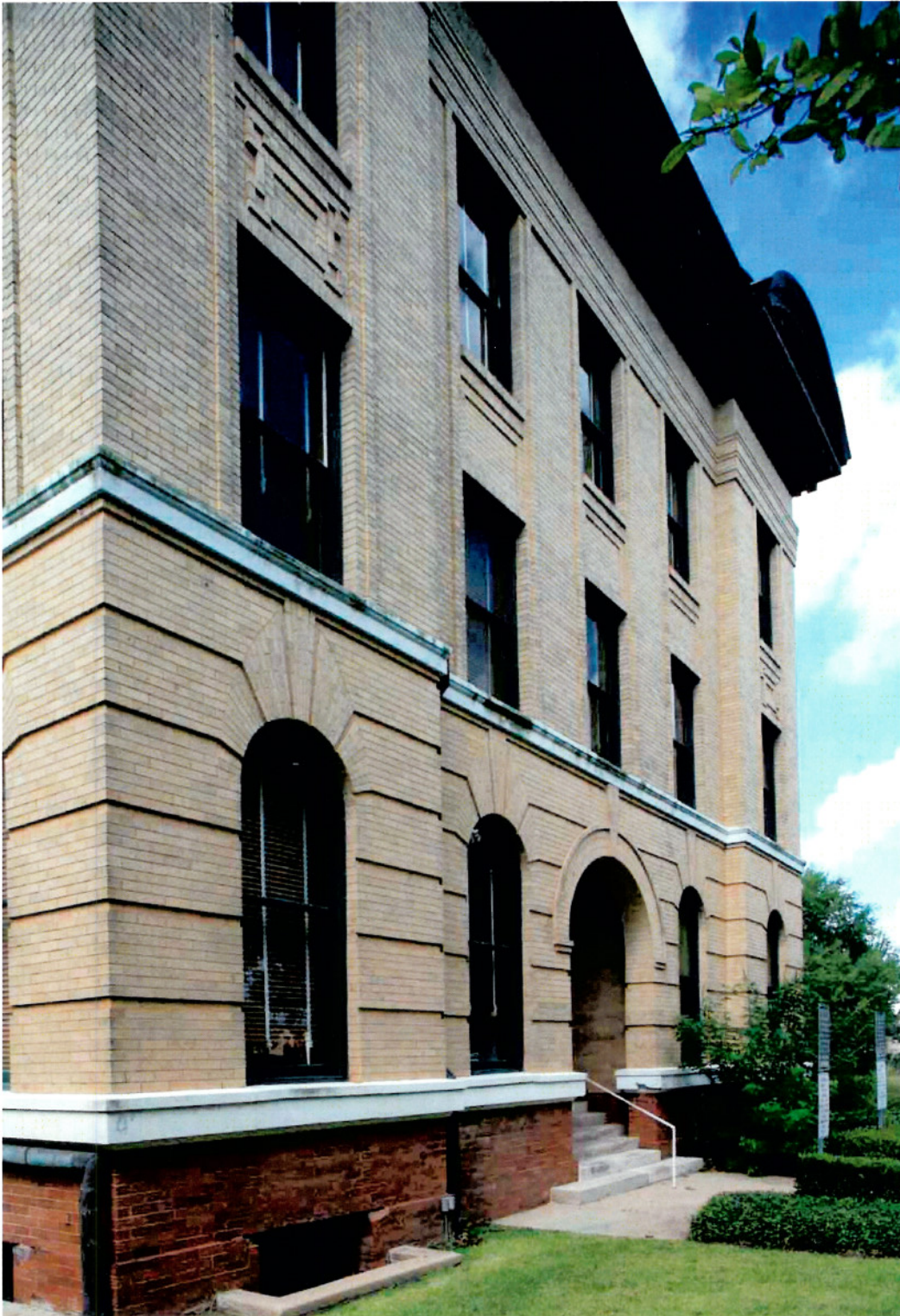
East Elevation, Masonry Problems: Settlement & Spawling at Basement Window, Displaced Water Table under Window, Poor Drainage at Second Floor String Course
