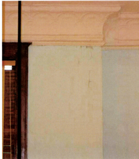
Rm 323: Water damage to wall from roof leak.
