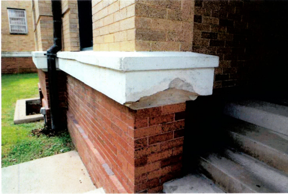
East Entrance: Broken cast stone water table where former handrail was attached.
