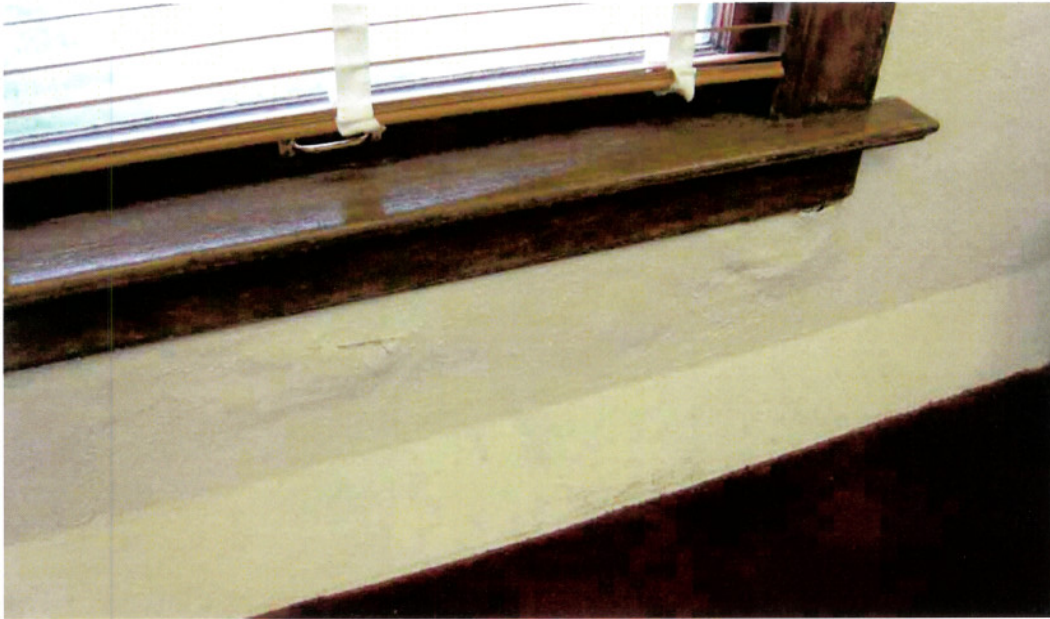
Rm 324: Water damage to plaster below window
