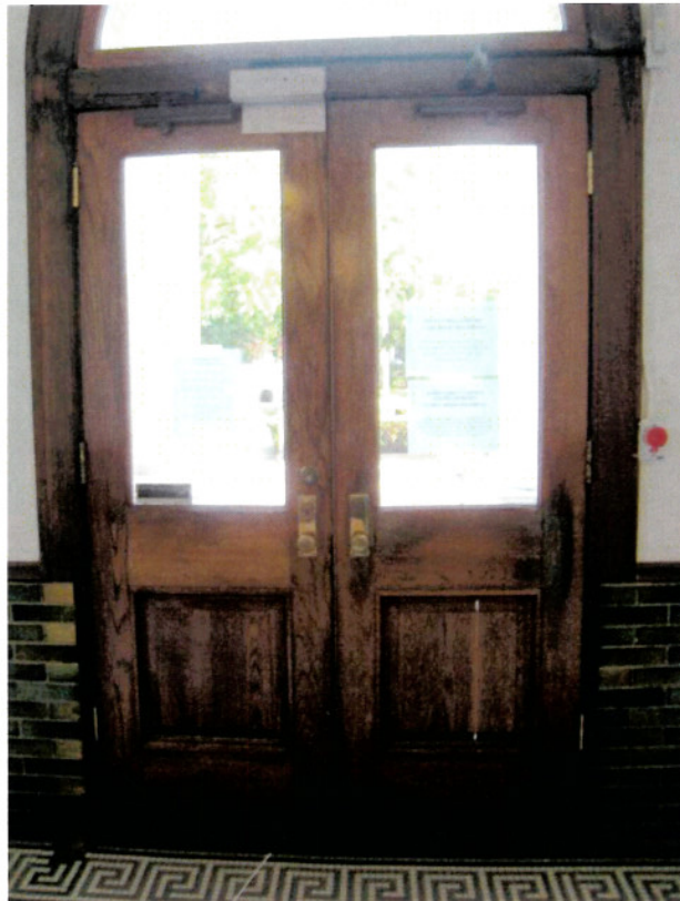
North entrance doors (not a public entrance) have severe mold at rails, cracked panels and are warped from magnetic locks.
