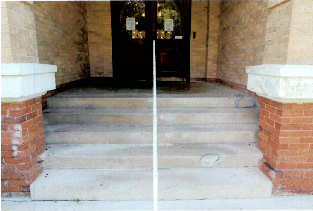
West Entrance: Broken Concrete Steps, Broken Cast Stone Water Table from previous handrail, doors severely cracked and no longer watertight.
