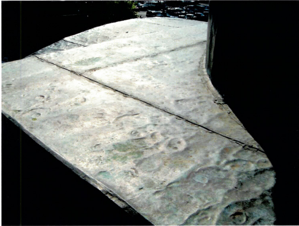
Deterioration of flat-work copper roofing at joints and penetrations; broken solder at seams, movement around anchors.
