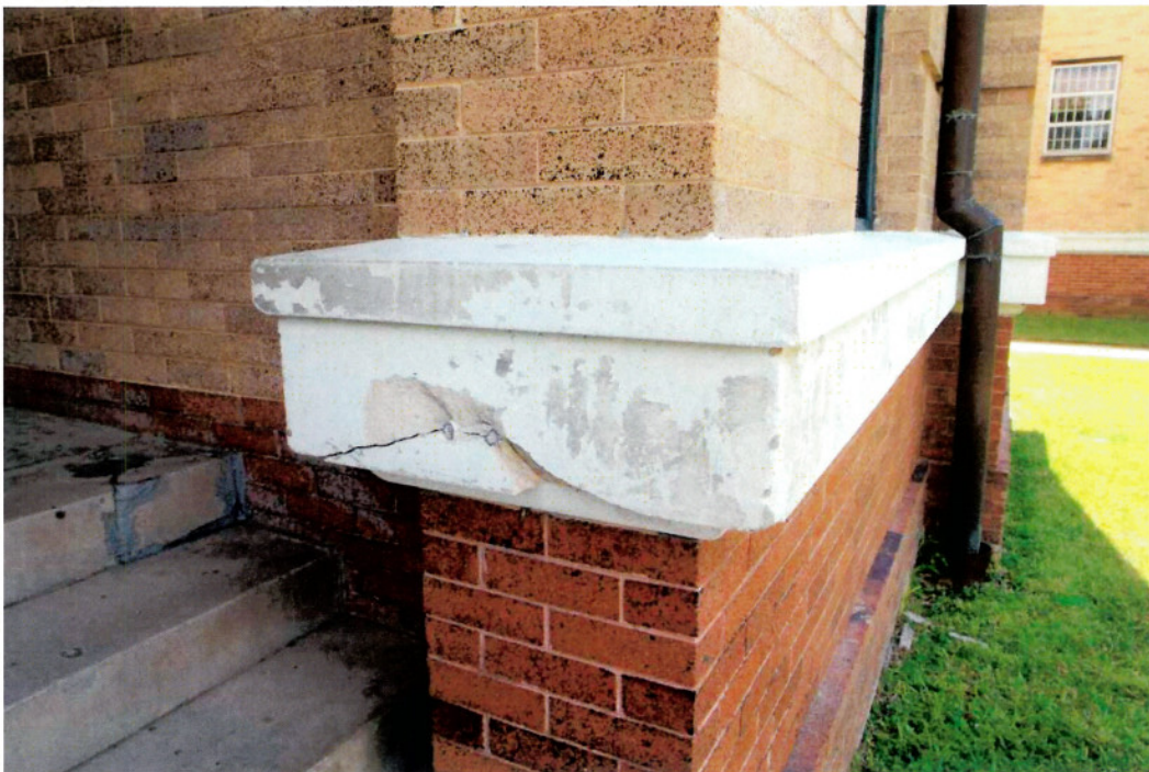
West Entrance: Broken concrete steps, broken cast stone water table where former handrail was attached
