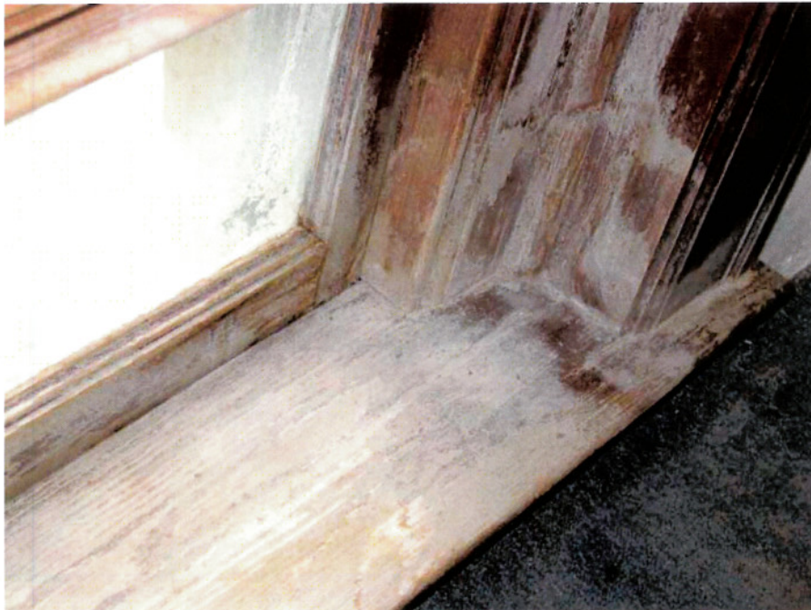
Rm 124: Deteriorated wood window & frame
