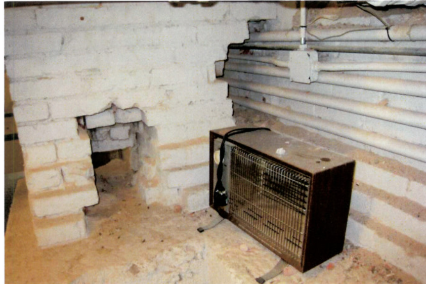
Foundation supports with large holes for current or previous piping.
