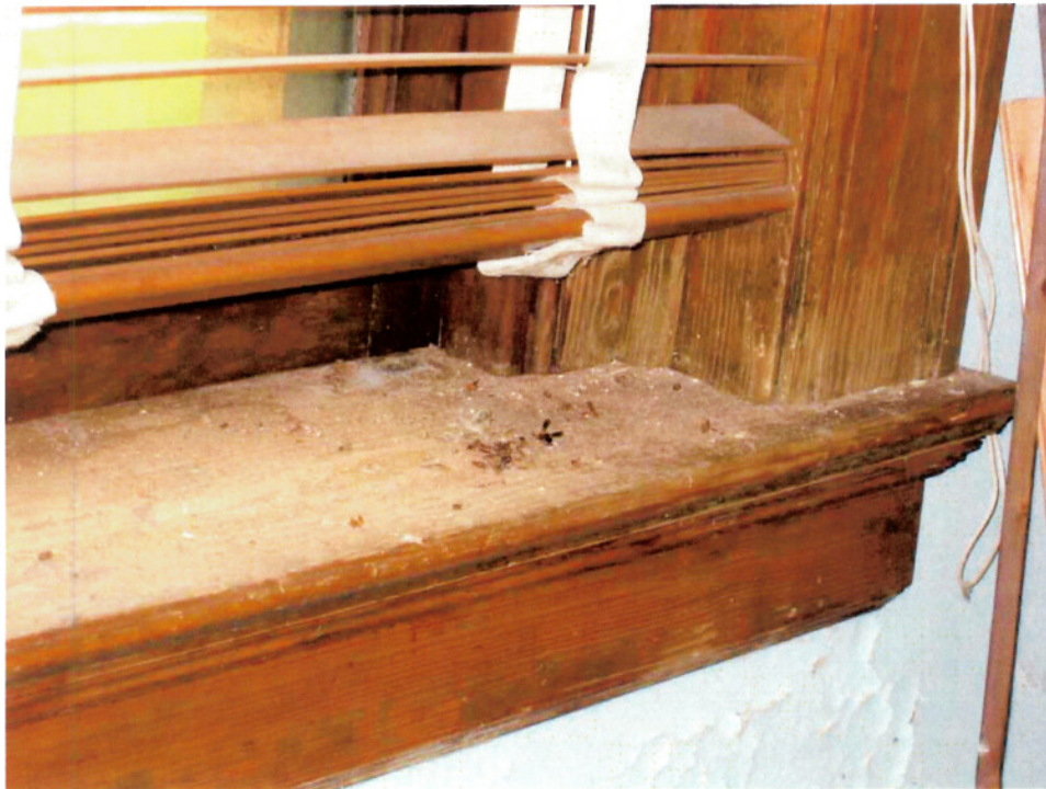
Rm 224: Deteriorated wood window & frame, evidence of termite infestation, plaster delamination below.
