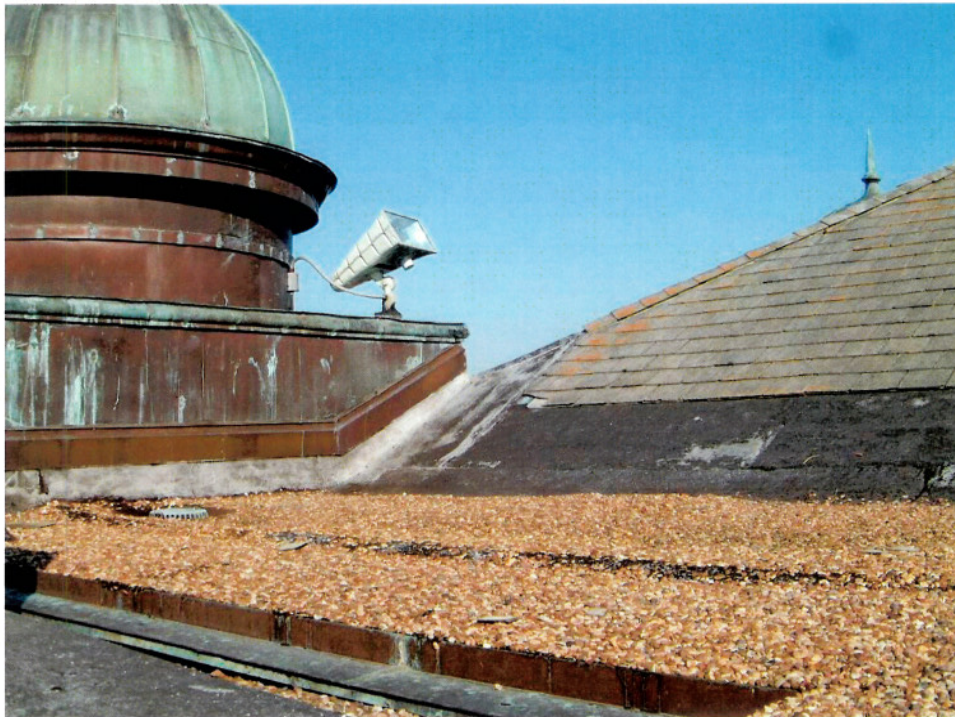
Roof deterioration; corroding and dissimilar anchors in copper, broken cement shingles, buckling BUR.
