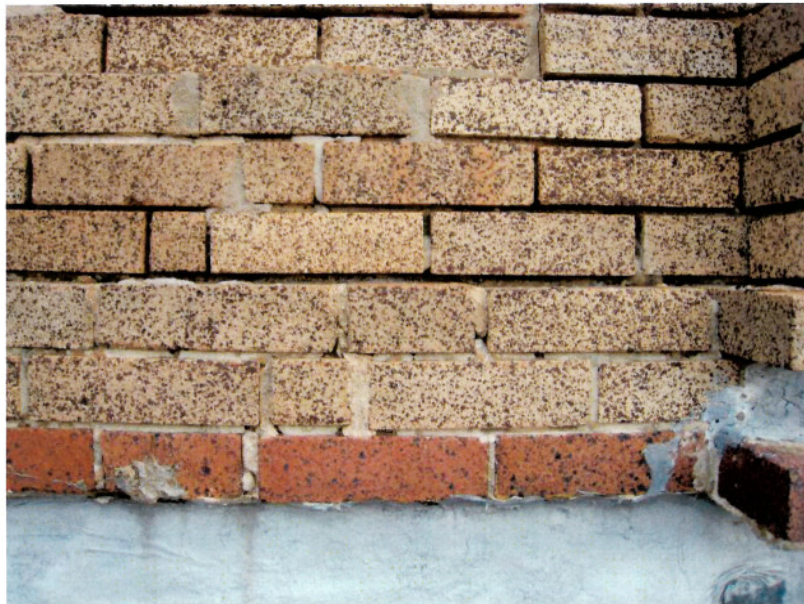
Deteriorated mortar at south wall parapet. Masonry is unsupported and falling to 1935 roof below.
