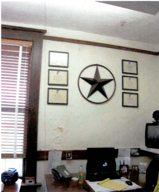
Rm 325: Water damage to ceiling & wall from roof leak
