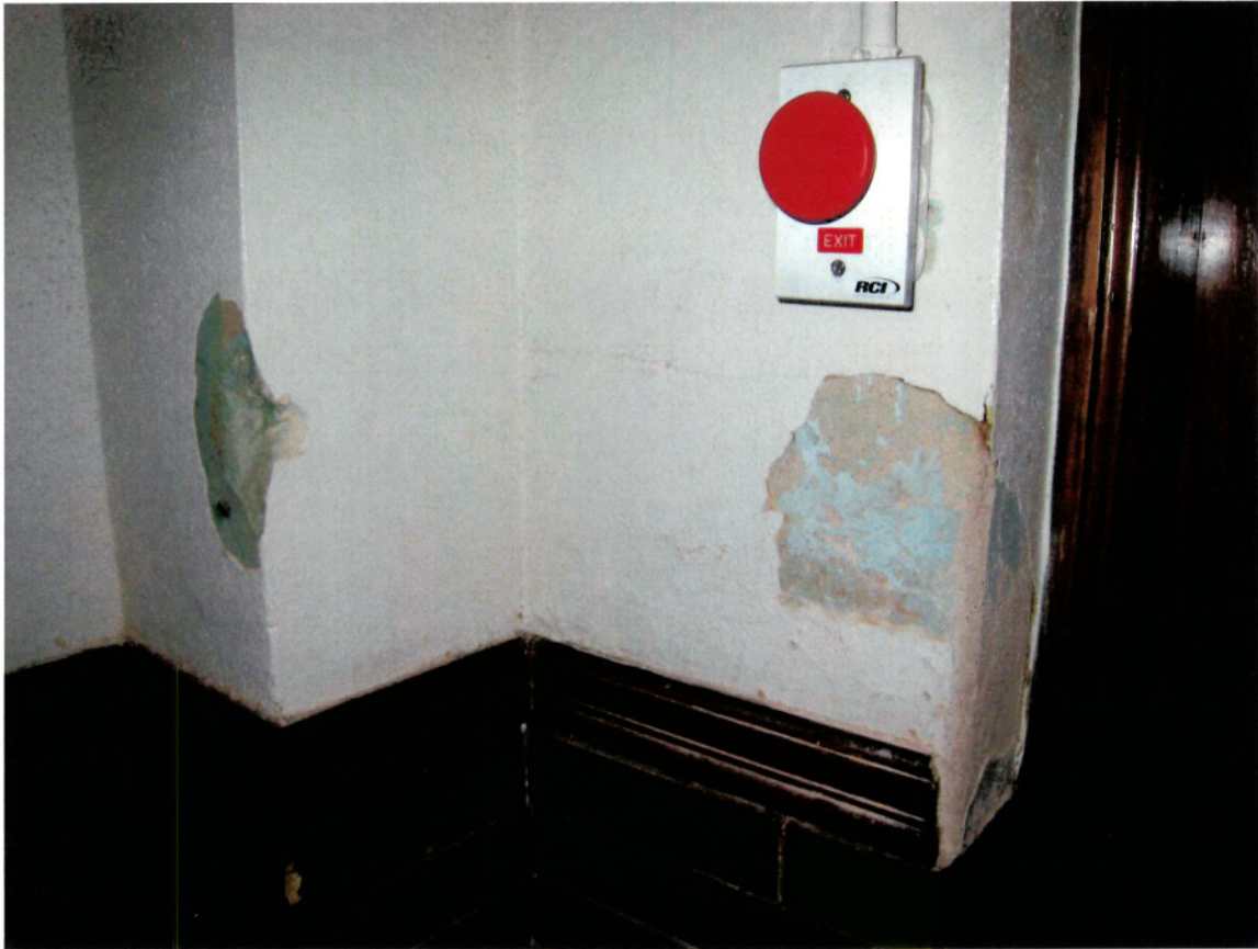
Interior plaster wall damage at exterior doors.
