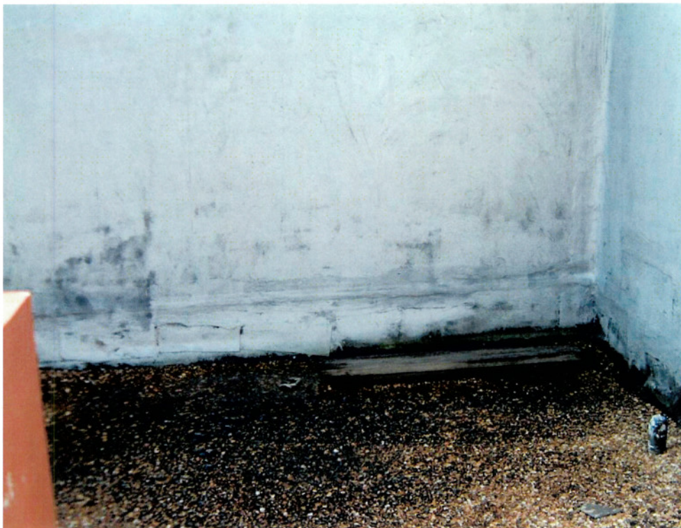
Deteriorated cant strip, standing water year round, clogged roof drain.
