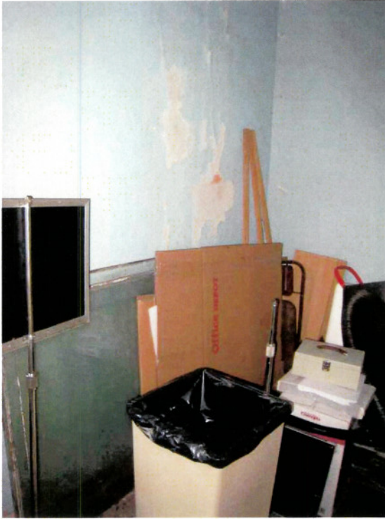
Rm 224: Water damage to wall, plaster delamination.
