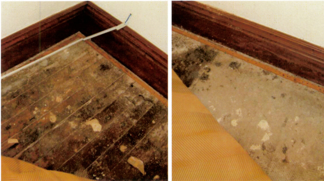
Mixture of original wood flooring (some with leveling compound) and concrete in same corner office.
