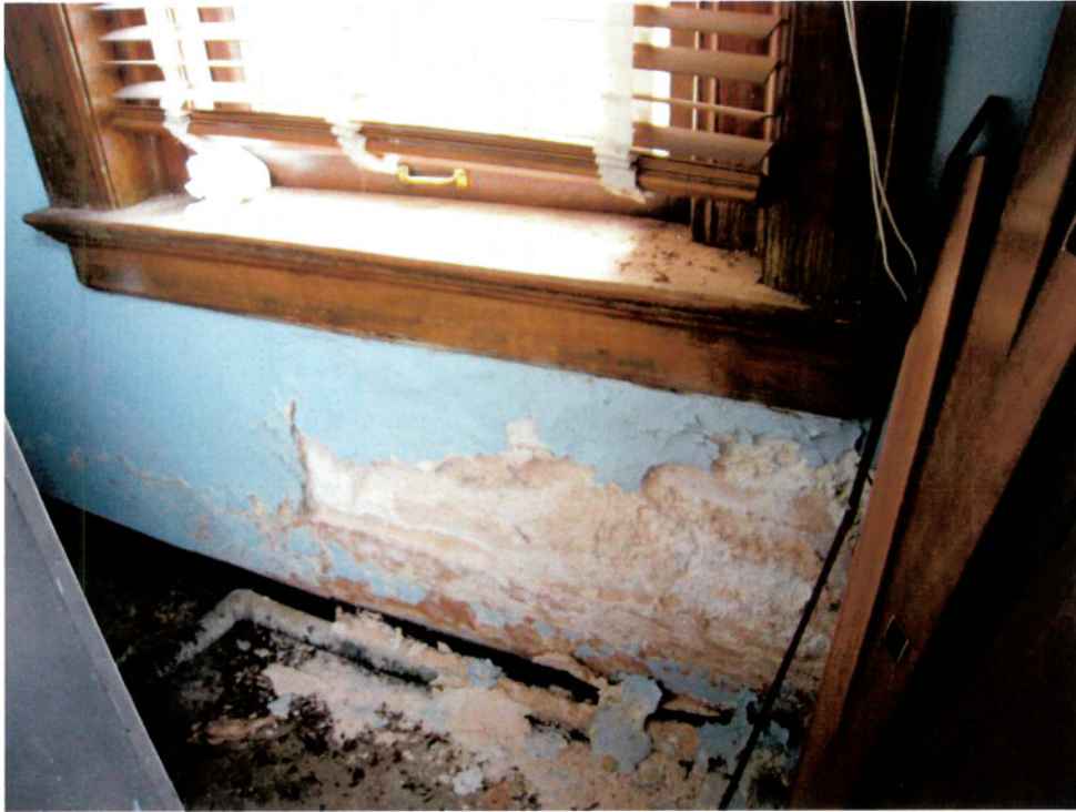
Rm 224: Water damage to wall beneath window at mechanical units, delamination of wall.
