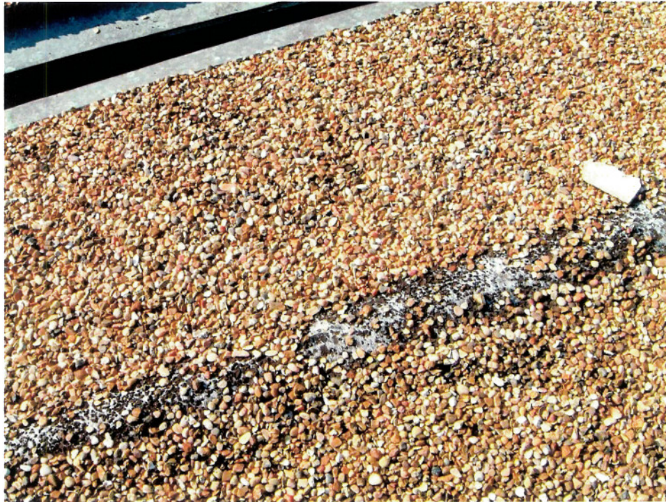
Bubbles in BUR indicate deck movement below or moisture collection
