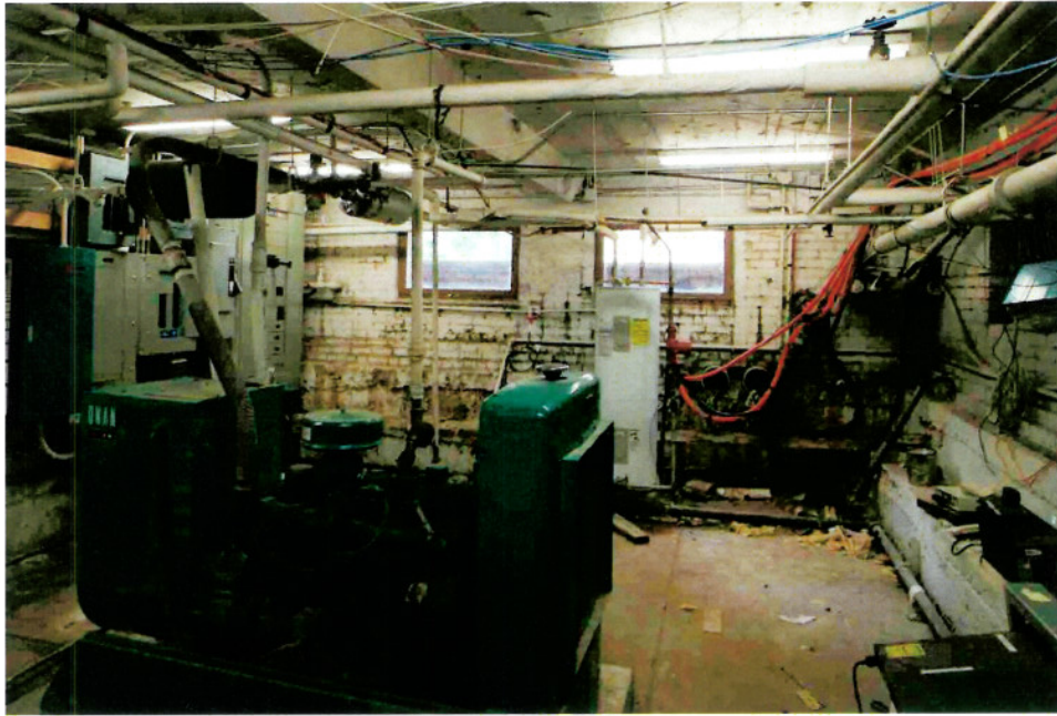
Rm 004: Generator, electrical panels, water heater located below grade and subject to flooding through basement walls. Mortar deteriorated from flooding through basement walls.
