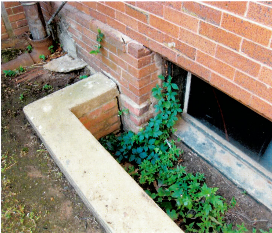
Light wells fill with water, water soaks through into basement deteriorating mortar, window lintels and wood windows. Light well shave separated from exterior wall.
